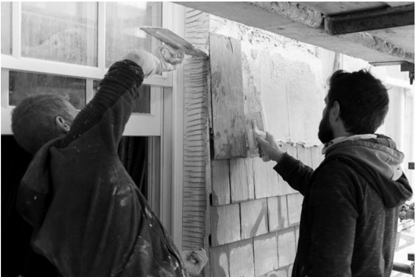
Hung slates being installed by Will and Mick of O'Brien and Donnellan Builders in 2021, by Andrew Campion Photography.
