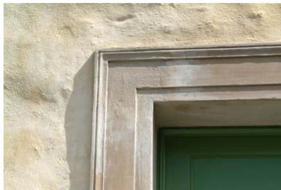
Lime harling with Shelter Coat on property in Kinsale, Co. Cork. (Naturally Hydraulic Lime also used to form reveal)
